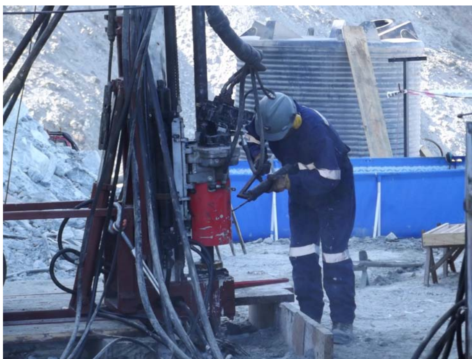
Current drilling on Platform B on which three diamond drill holes will be drilled to test a section of the target Cu-Au mineralised breccia.
